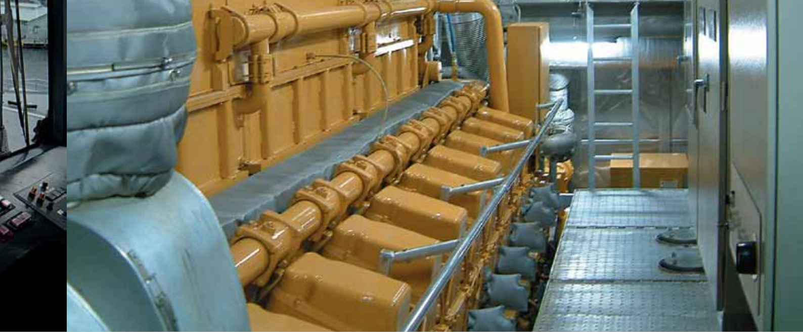
Caterpillar Generators on Hull 061
